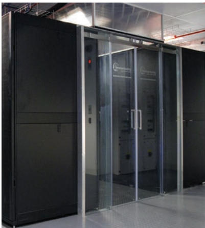
The new facility has 6,000ft 2 of technical space across two data halls, and features separate dual A+B power feeds to each rack.
