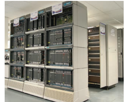
Comtek says it's able to repair and service equipment that has long been out of production, including the complete range of Nortel products such as the DMS 100 switching equipment shown here.
