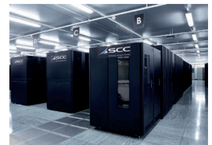
SCC will provide the council with a variety of services including data centre hosting.
